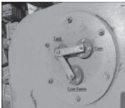
Fig.2: Earthing of Tank, Core and Core frame on the top cover of the transformer.
