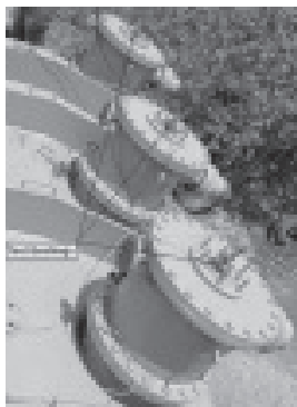
Fig.3: Epoxy test bushings and test leads connected to them for LT tests on the Trailer.
