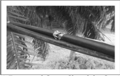
Figure 6: Damaged Outer Sheath by Squirrel Bite
