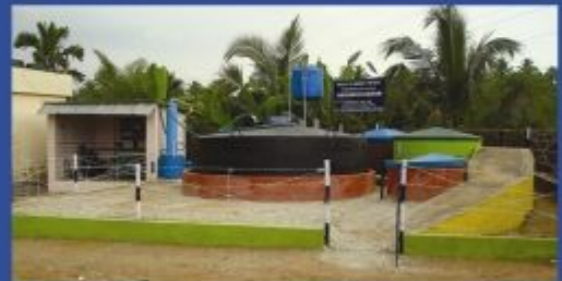
Waste to electricity plant
