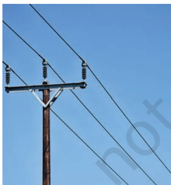
Fig. 4.54 Low Tension Distribution Lines (LT)
