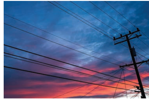
Fig. 4.50 Power Distribution Lines
